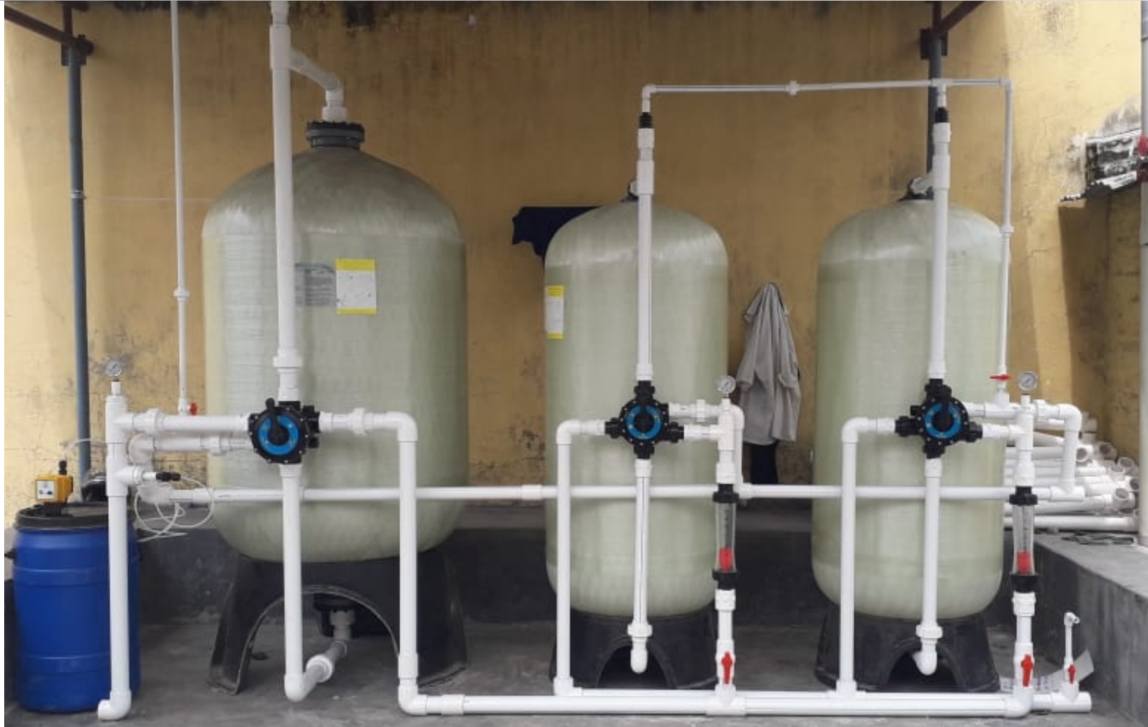
Iron Removal Plant Katihar - Bihar
